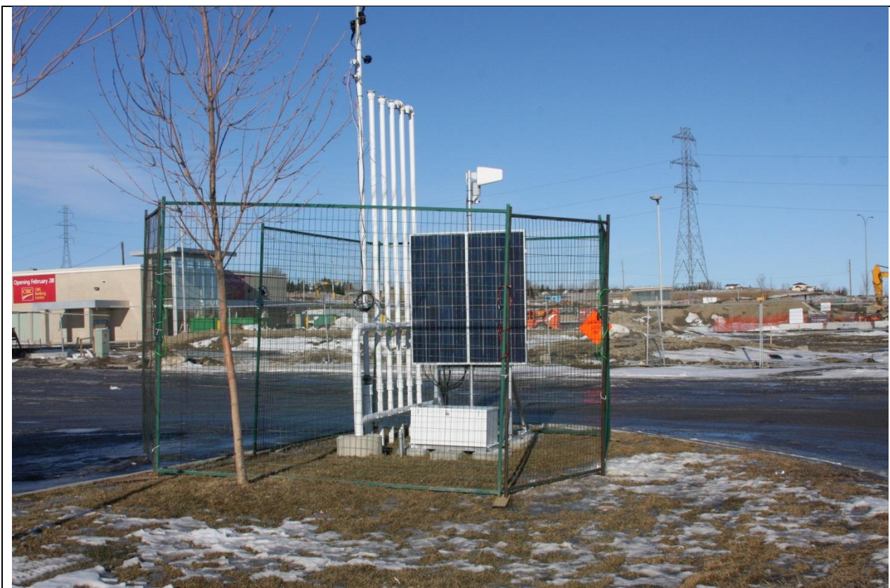
Figure 12: Photograph showing the temporary solar-powered vent emission monitoring system (VEMS) installed to monitor evaporation losses from an underground gasoline storage tank.
