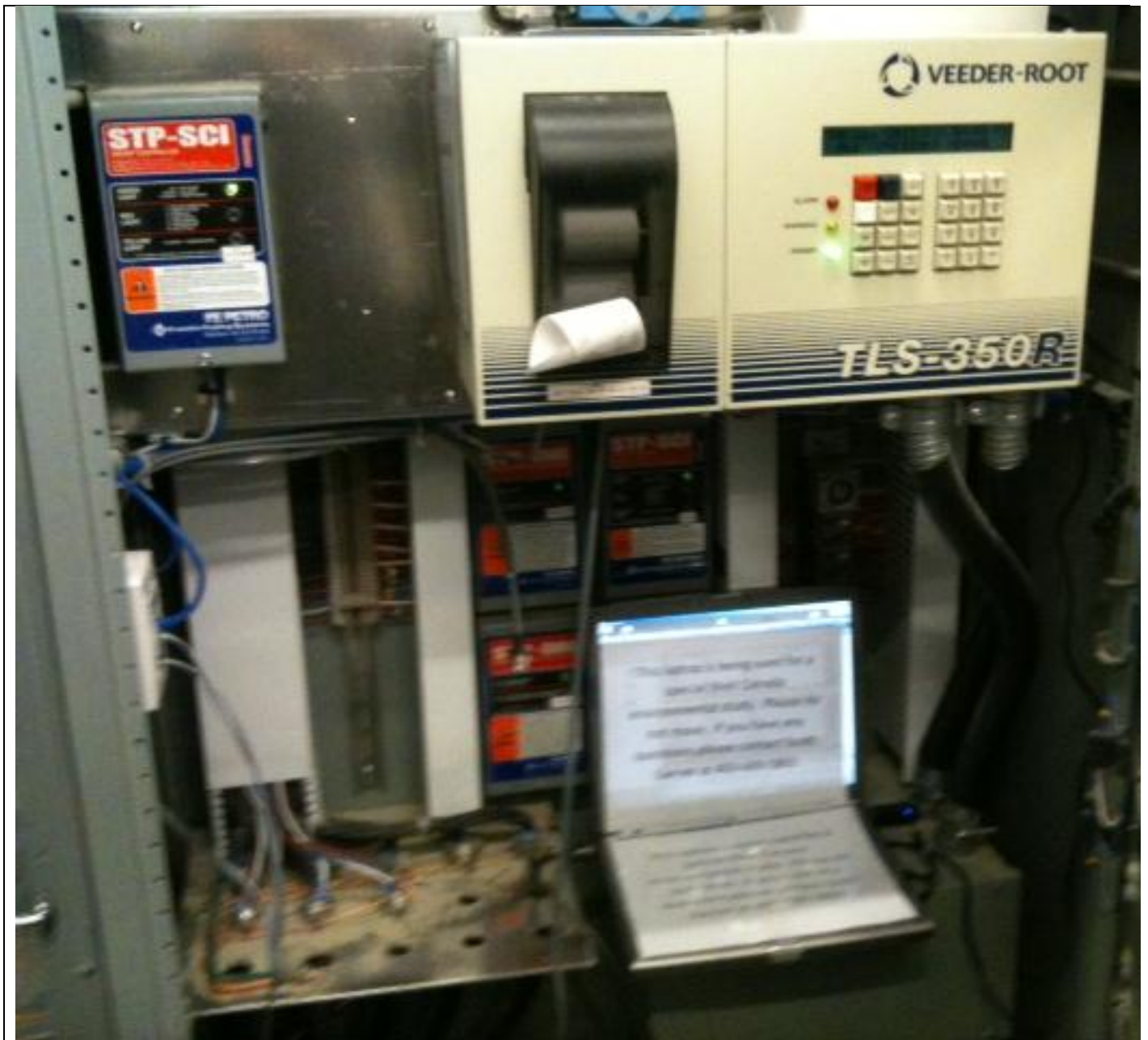
Figure 8: Photograph of the backroom control and data acquisition system for the Veeder-Root automatic tank gauging and leak detection system.
