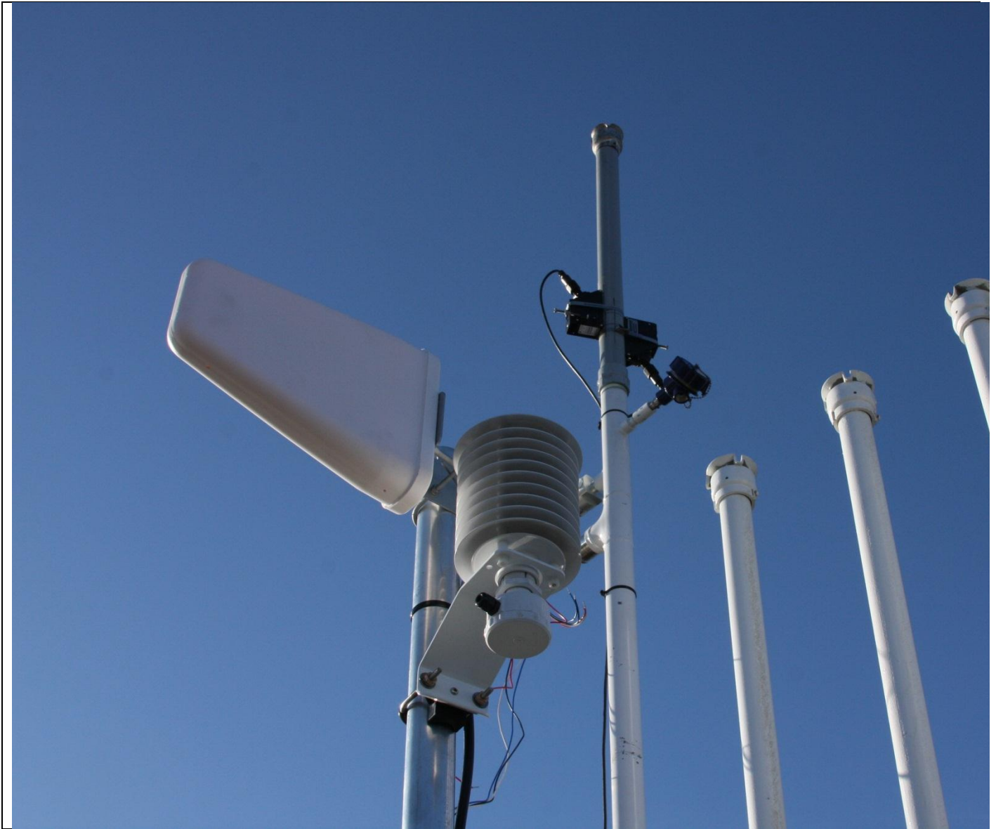
Figure 9: Photograph showing the ambient temperature and relative humidity sensor.
