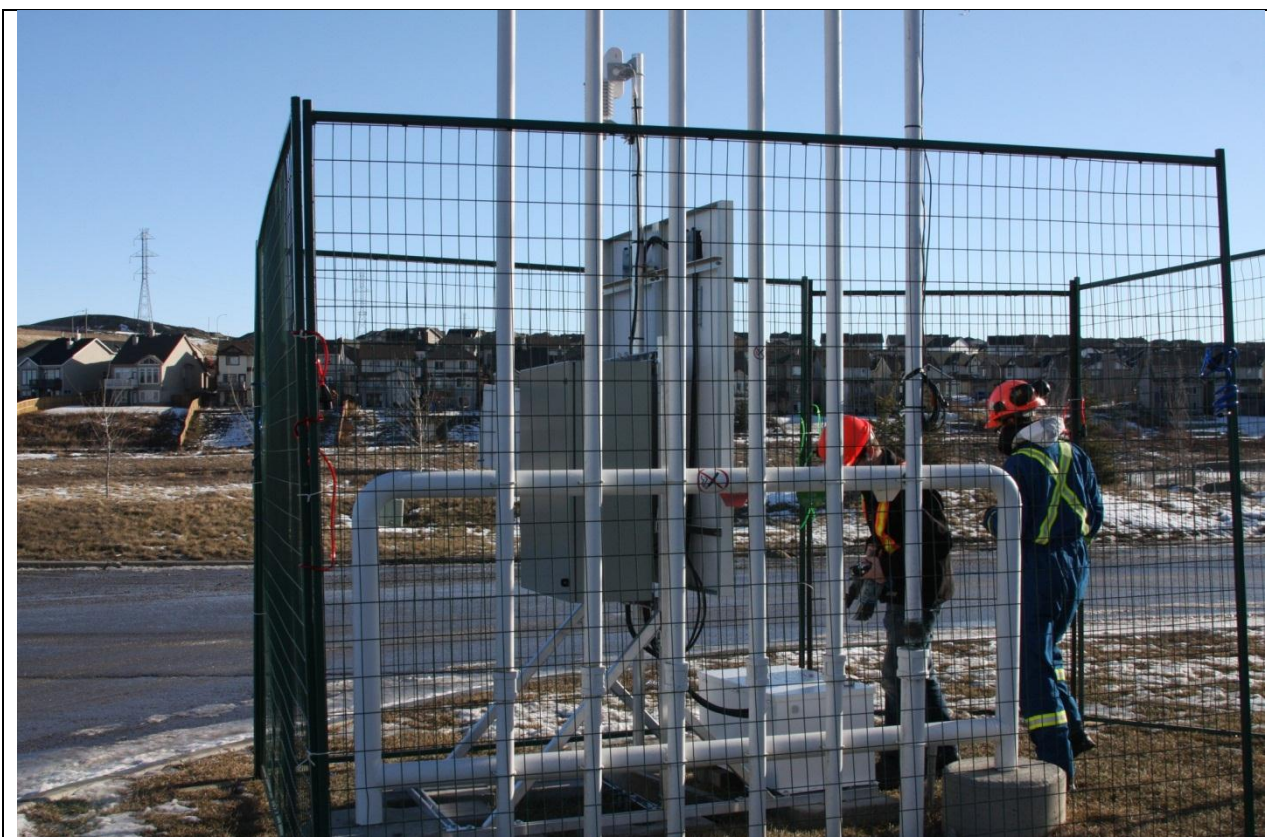
Figure 13: Photograph showing a different view of the temporary solar-powered vent emission monitoring system (VEMS) installed to monitor evaporation losses from an underground gasoline storage tank.
