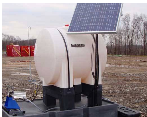
Figure 2: Solar chemical pump installed south of the 49 th parallel
